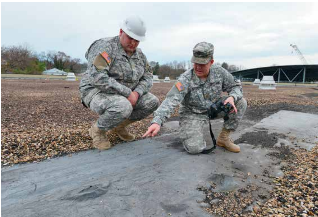
Stephen Finlon '16 and Maj. Paul Ackerman '93 inspect the Cameron Hall roof. – VMI Photo by Kelly Nye.
